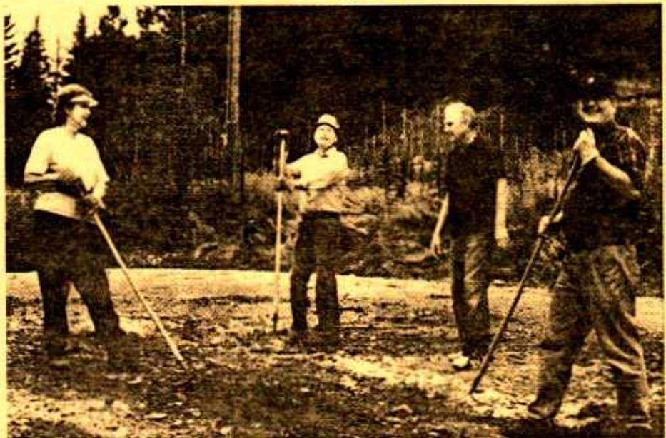
Part of the crew that worked on the Fishermans Lane cul-de-sac. From left are Verna Heidebrecht, Jack Heidebrecht, Charles Heidebrecht and Guy McCoy.
