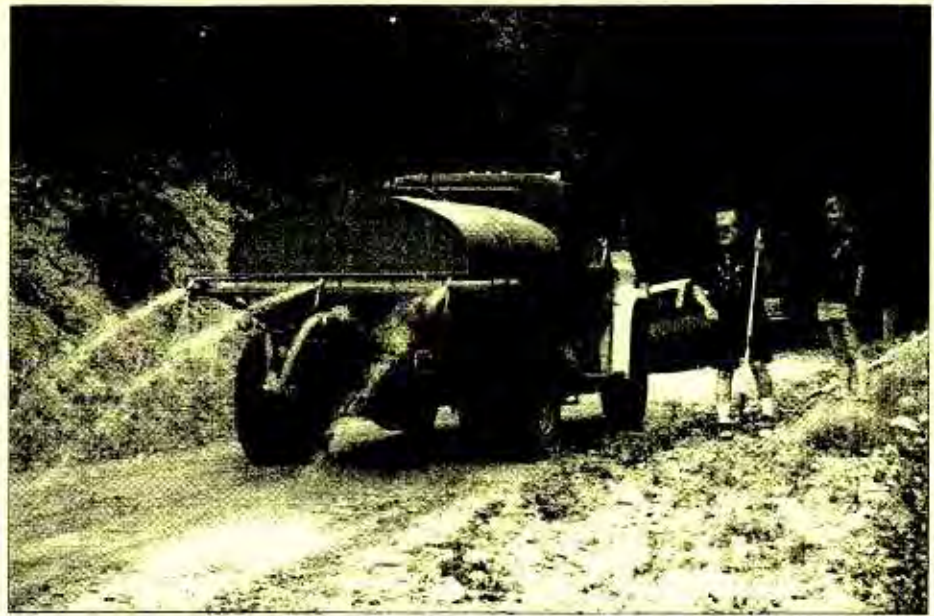
Steve and Irene Little prepare to rake newly applied recycled asphalt after Al Cunningham finishes spraying it.
