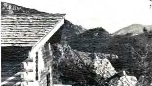
First cabin constructed by Terrino (tract 96, F.1) nears completion. The view faces east.
