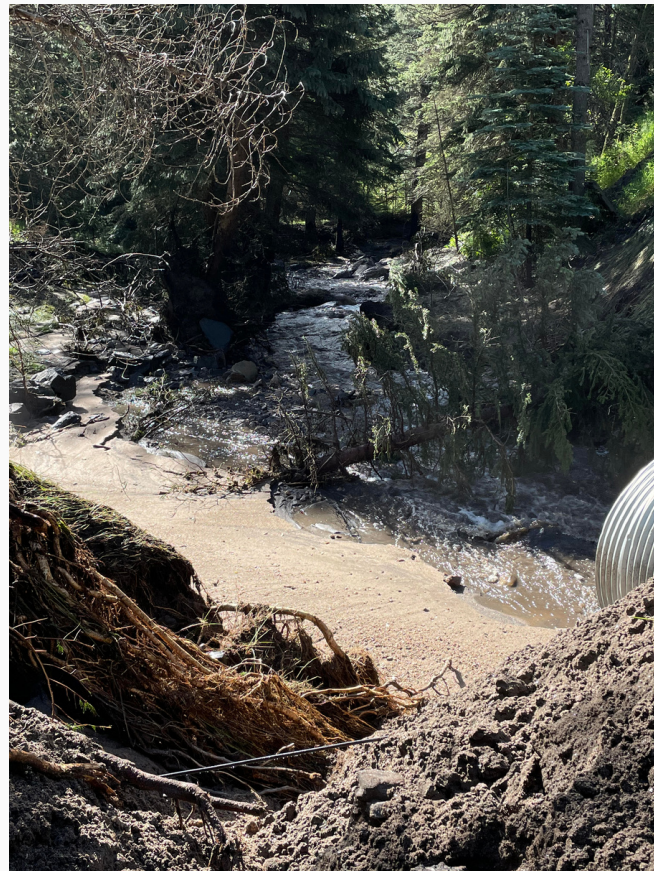
Flood damage Miller Fork Culvert 7-15-22
